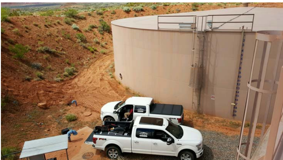
SCADA Integration in Ivins, UT
